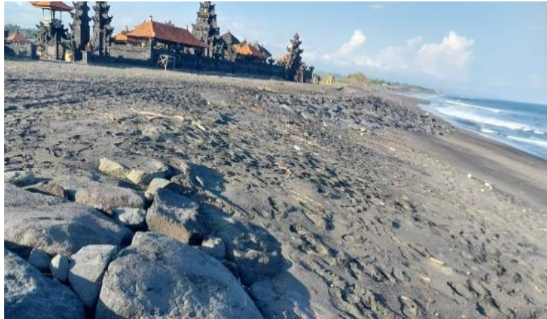
Figure 1. The condition of the revetment at Rangkan Beach
